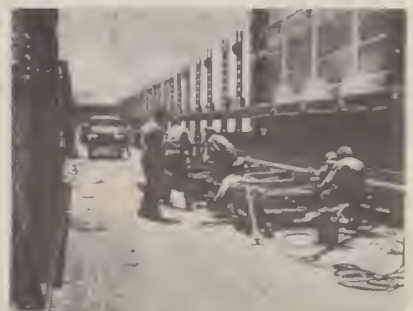
An outer truss unit on the north roadway is assembled for erection against the Manhattan tower.
